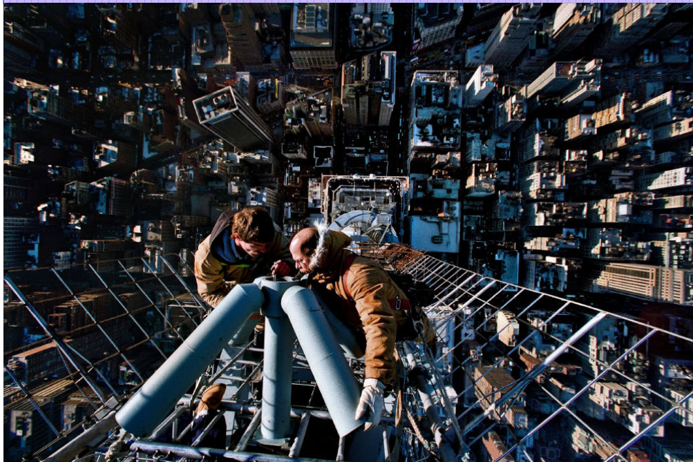
Specialists make adjustments to a television transmitting antenna atop the World Trade Center
